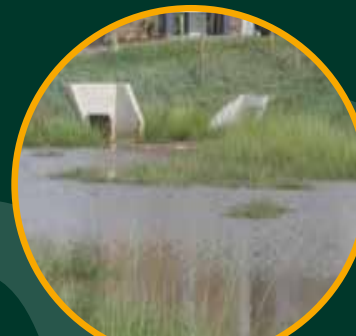
Shallow attenuation basins
