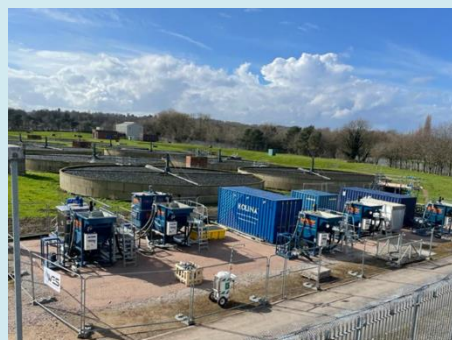
Figure 6: Our alternative P removal test bed at Woolton WwTW
