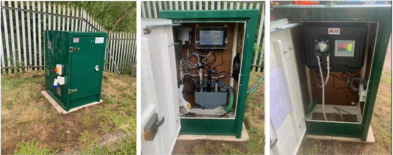
Figure 21: Continuous river monitoring - Kiosk based solution pilot in Cheshire
